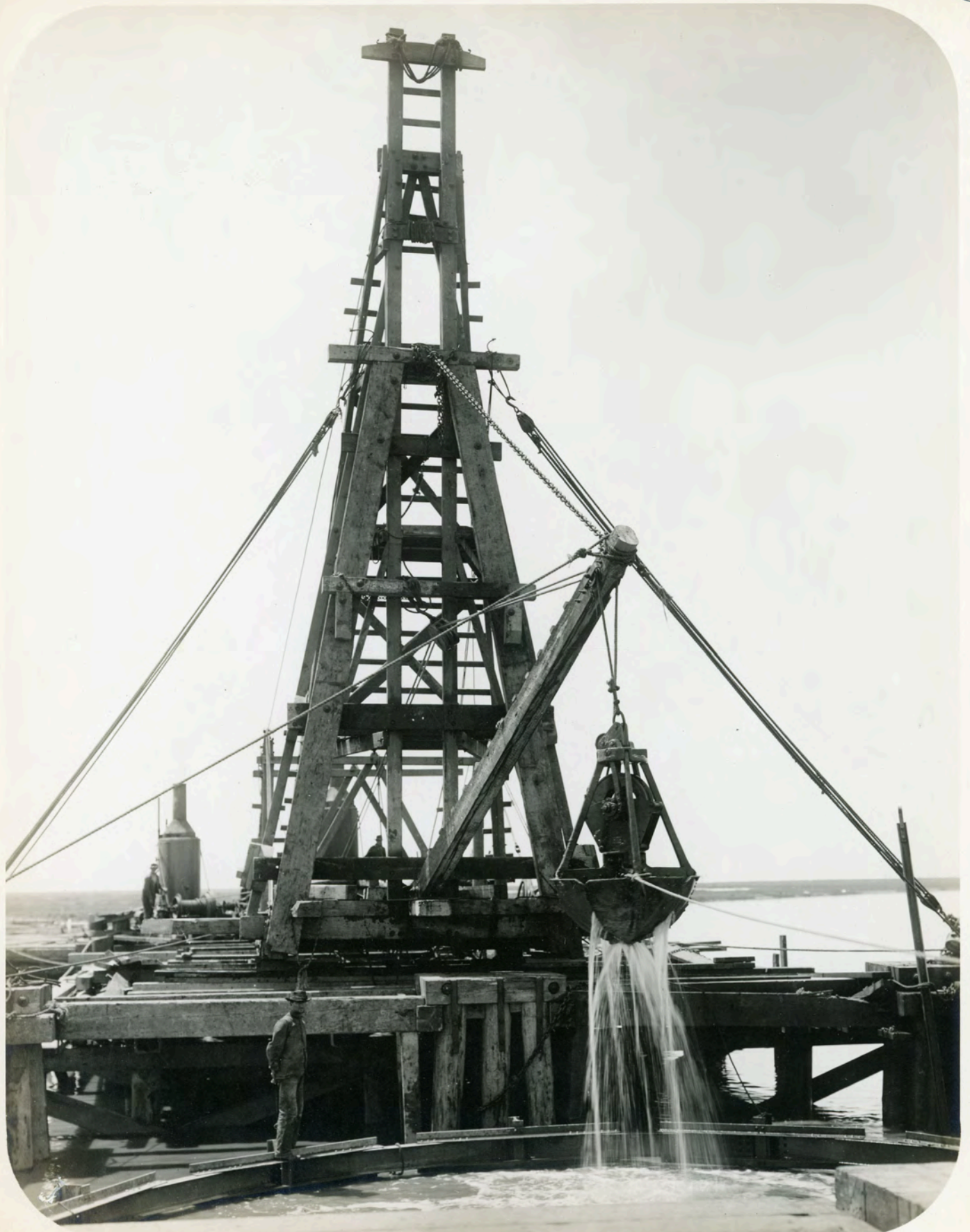
CEN. CAL. Ry. Dredging inside of Casing for Pivot Pier, Newark Sl. Draw. June 12, 1908
