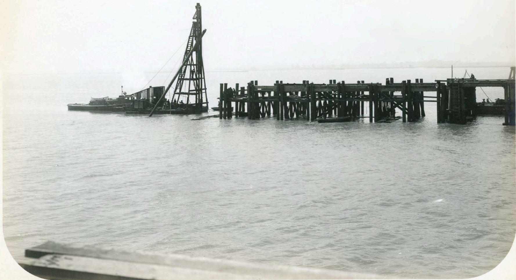
CEN. CAL. RY. Driving piles for Protection of Bridge, Dumbarton Pt. Draw. Aug. 18, 1908.
