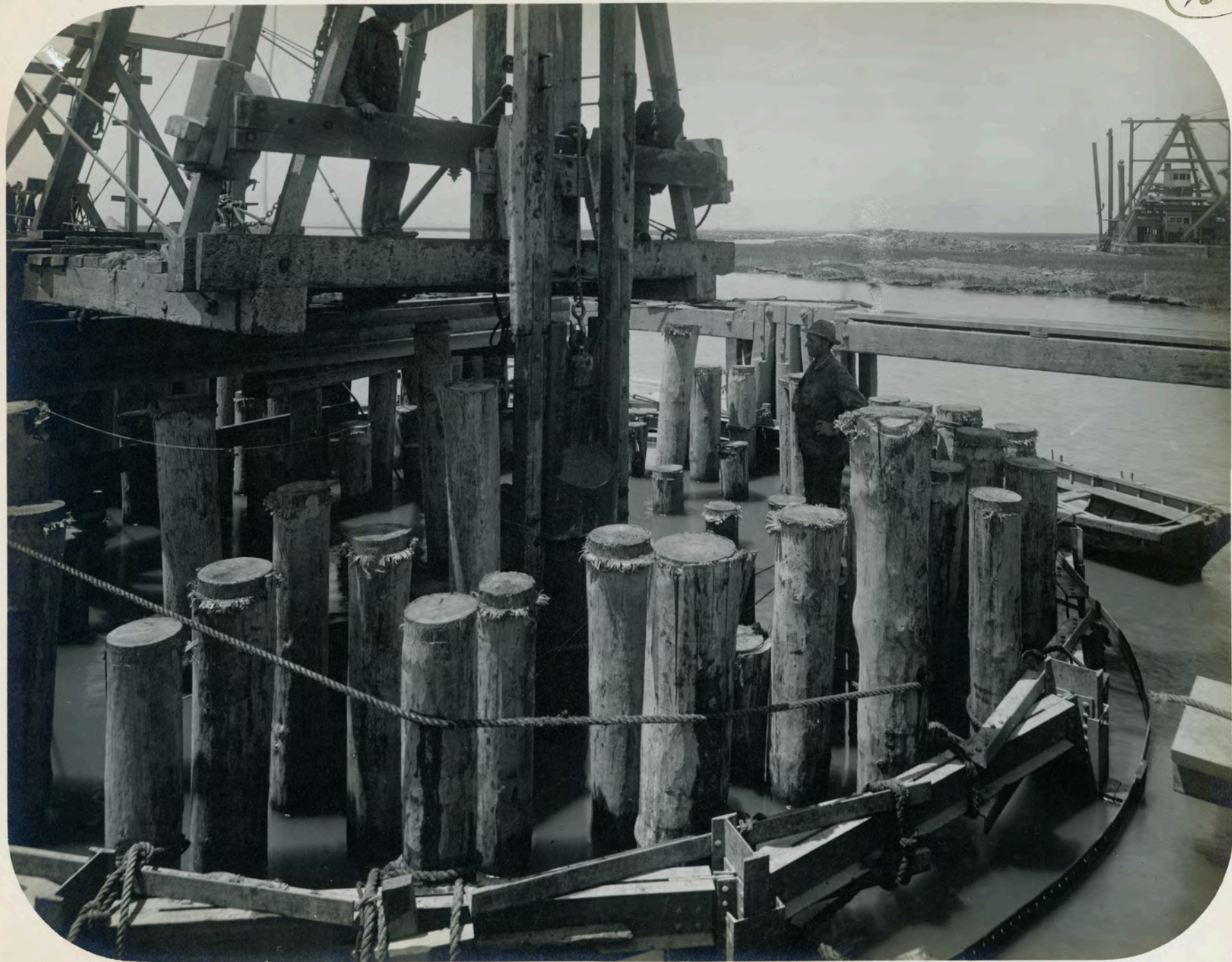
CEN. CAL. RY. Driving Piles inside of Casing, Pivot Pier, Newark Slough Draw. June 24, 1908
