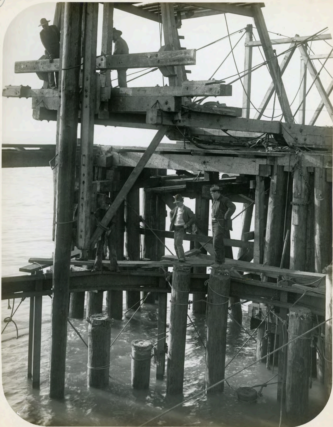
CEN. CAL. RY. Driving Foundation Piles for Pivot Pier, Dumbarton Pt. Draw. Nov. 16, 1908.
