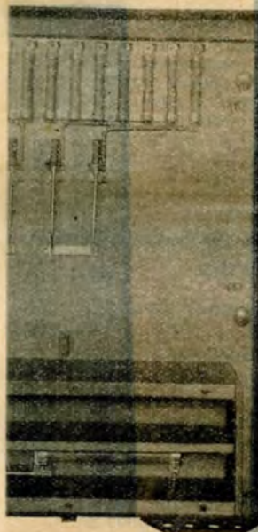
Switchboard, Control Car
