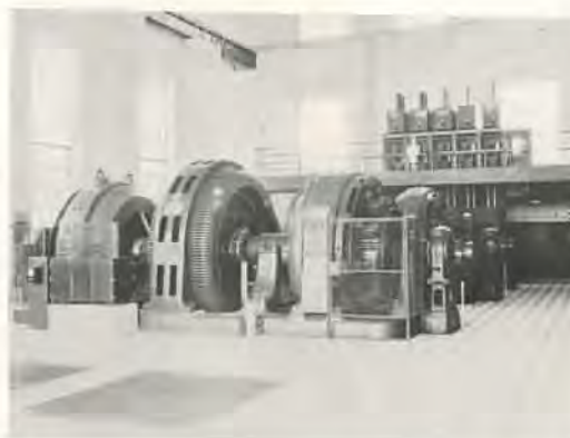
Interior of Maltrata Substation
