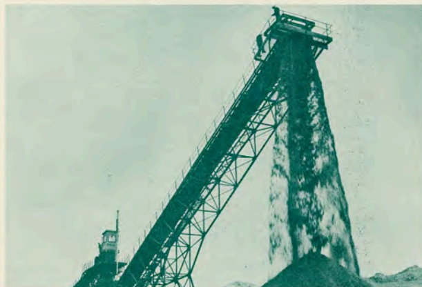
● At the end of the conveyor system a cascade of gravel pours onto the storage pile near the barge loading dock.
